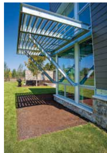
Shuttered awnings allow for passive solar heating in the winter while providing shade in the summer.
