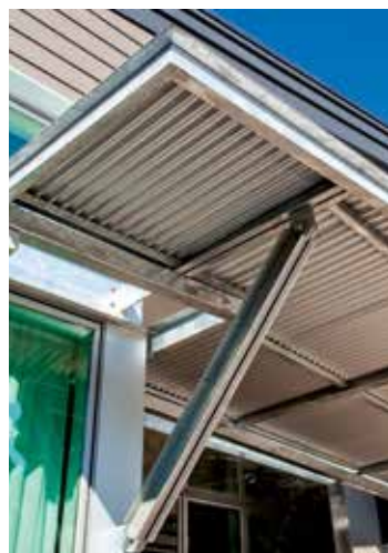
A corrugated steel awning above the main entry mimics window treatments elsewhere on the exterior.
